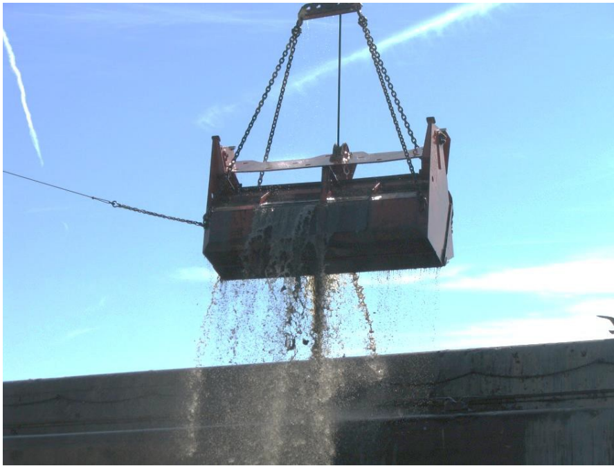
Figure 2. Fourteen cyd closed environmental bucket used by the Dredge DB Palomor in the Port of Richmond.
