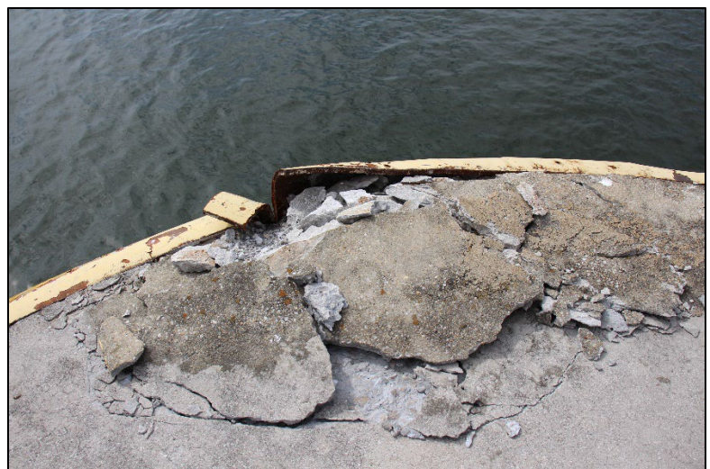
Figure 2. Crushed concrete on the bullnose of the upstream guidewall at Wheeler Lock.
