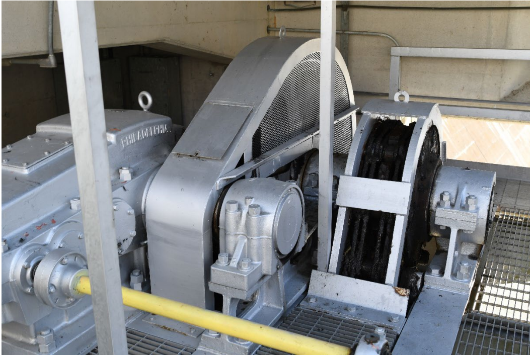
Figure 2. Close-up of existing lift chain equipment at the Cordell Hull Dam.
