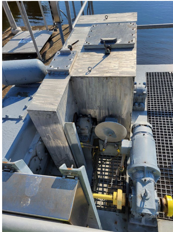
Figure 3. Overview of cable lift equipment at the Calcasieu Saltwater Barrier.
