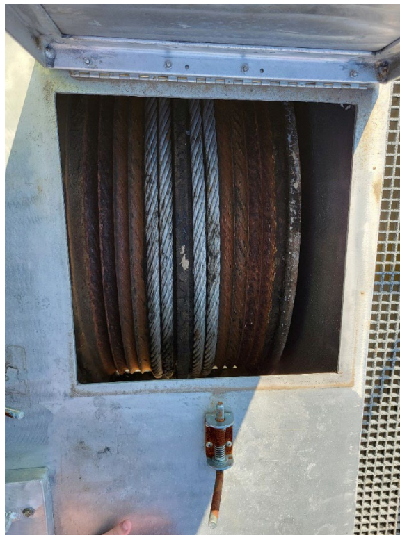
Figure 4. Cable drum at the Calcasieu Saltwater Barrier with provision for 6 winds of dual 1.25-in. cables.
