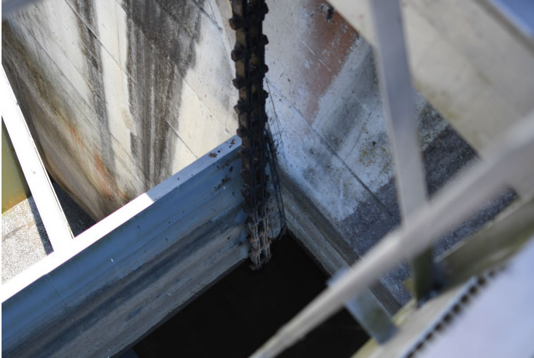
Figure 5. Chain interfacing with the gate at Cordell Hull.
