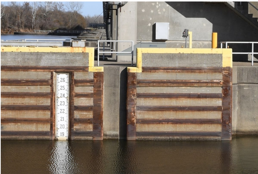
Figure 4. Existing 55-ft. bulkhead slot on the upstream, river side monolith at Emmett Sanders Lock and Dam (Lock 4).
