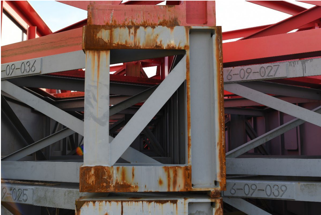
Figure 3. Corrosion on 55-ft. bulkheads in storage on the bank of the Arkansas River.
