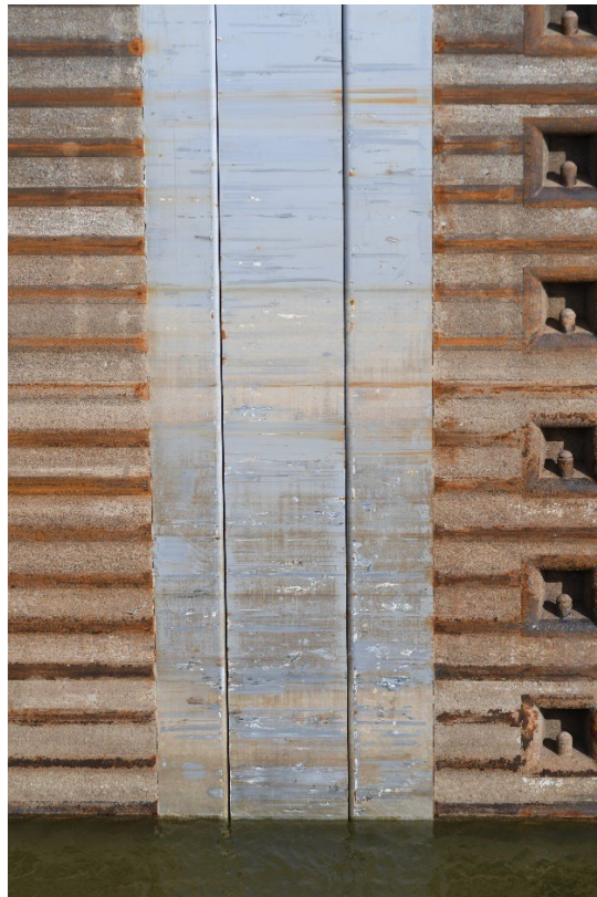
Figure 6. Frictional wear primarily on the lower portion of a bulkhead slot protection plate at Norrell Lock and Dam (Lock 1).
