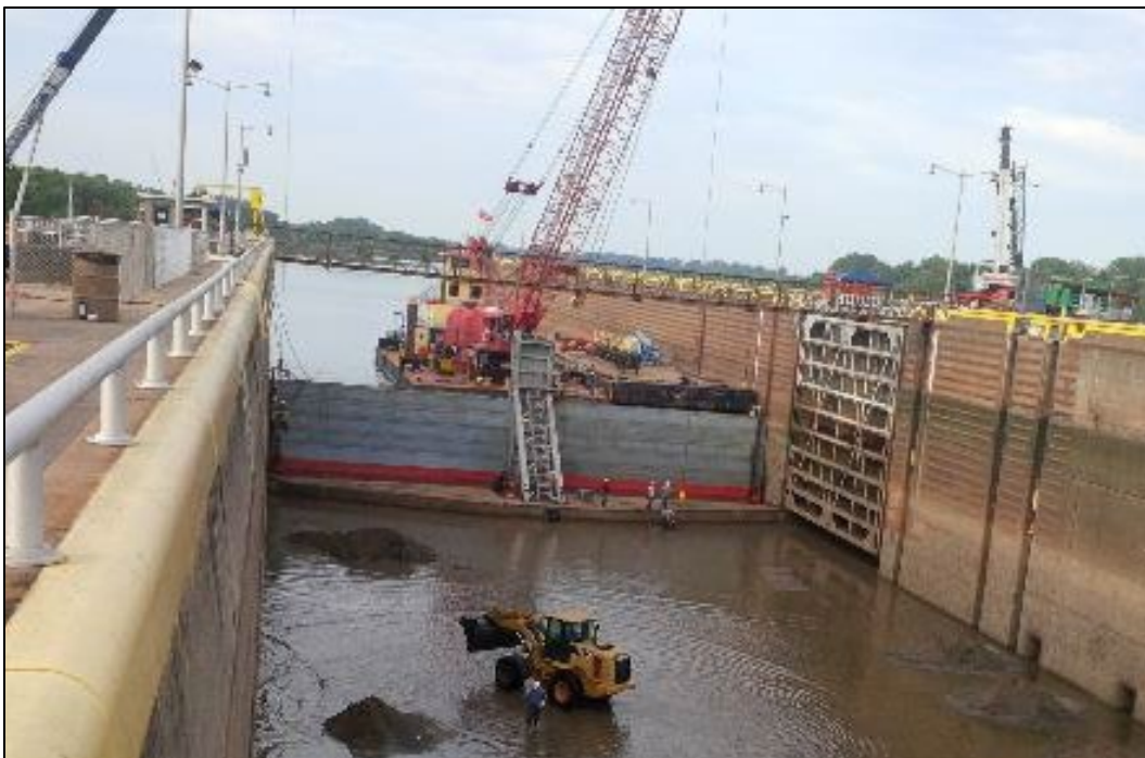
Figure 1. Example of 55-ft. bulkhead and center post system in service.
